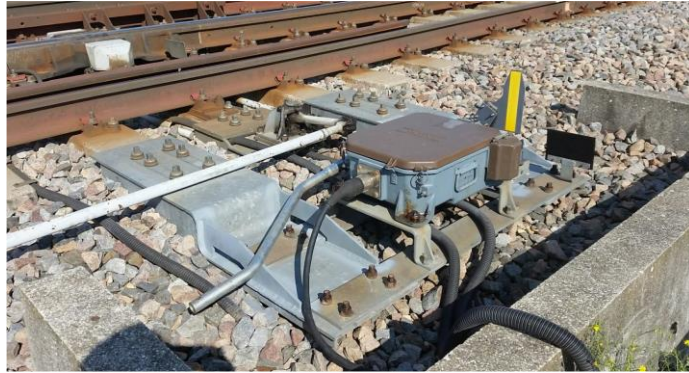
Figure 1 Picture of support and switch engine box actuating the point blade, clamped to sleepers and partially supported by ballast
