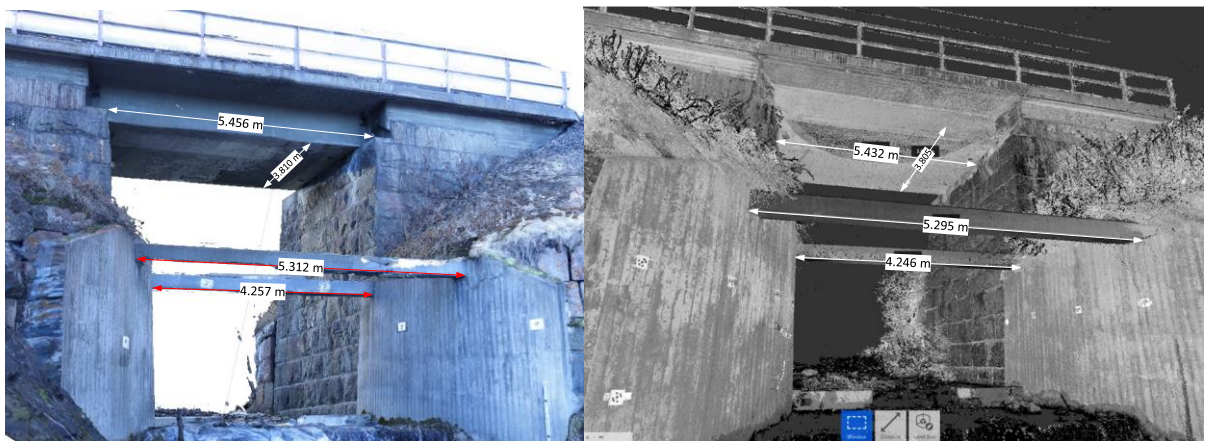
Figure 4: Measurements of bridge structural elements in both CRP (left), and TLS (right) method
