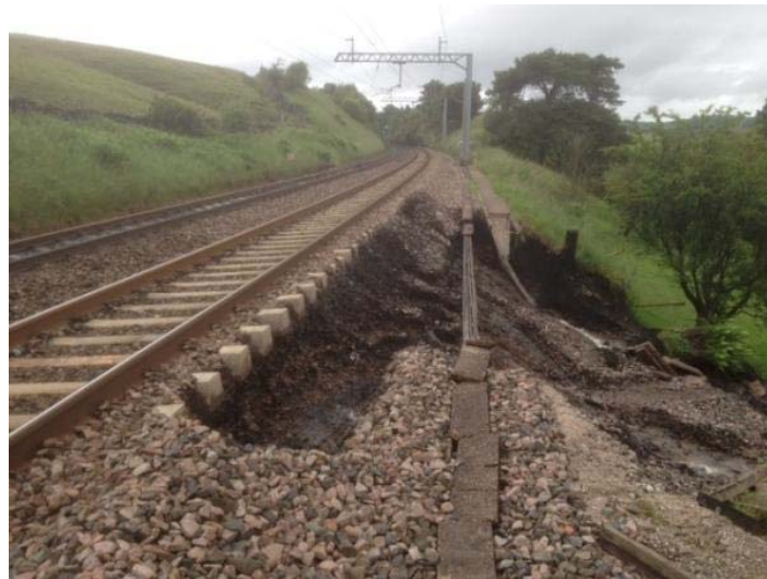
Figure 2 UK Slope failure (courtesy T. Morgani)
