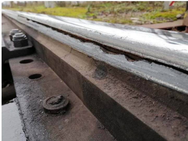
Figure 1: Heavily worn switch rail with characteristic break outs.
