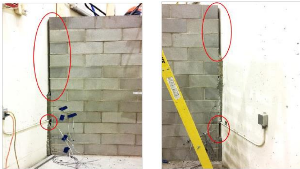
Figure 5: Loss of bond experimentally observed [4].
