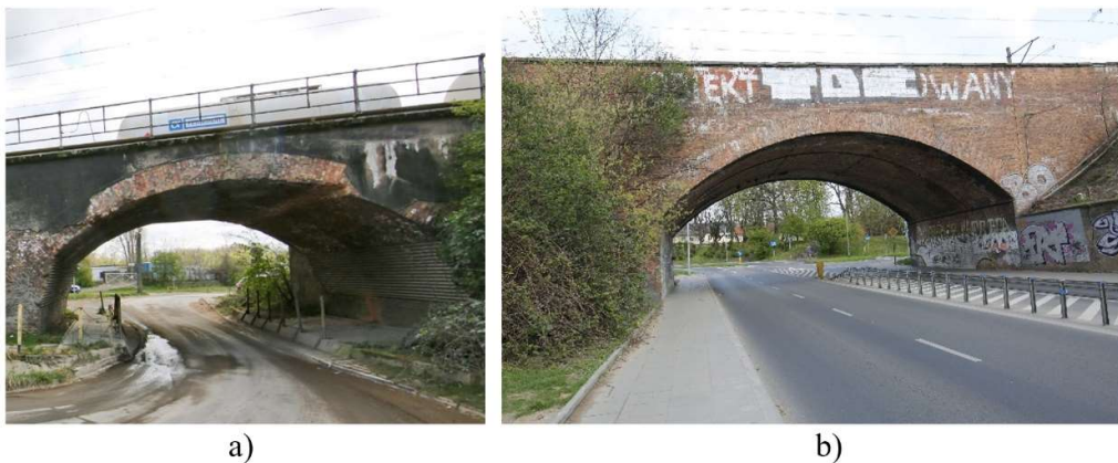
Figure 1: The analysed bridges: a) over the Fabryczna street, b) over the Wilcza street.
