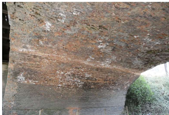
Figure 6: Intrados damage of Fabryczna Street bridge.
