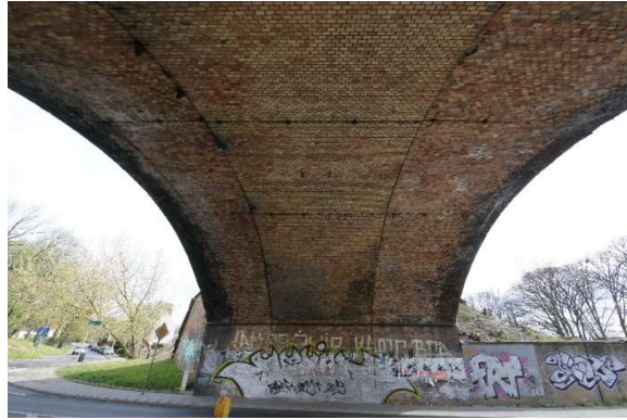
Figure 7: Intrados damage of Wilcza Street bridge.
