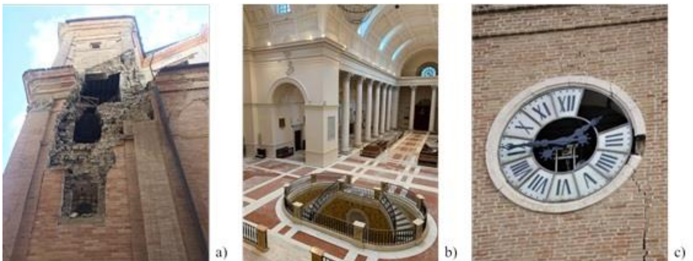
Figure 4: Some cracks after the Central Italy Earthquake, a) Partial collapse of one façade side of Santa Maria in Via; b) Cracks spread on the walls and the vault of San Venanzio; c) Crack in correspondence of the Clock of one Santissima Annunziata bell-tower.
