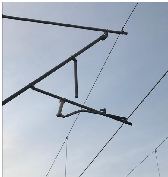
Figure 2: Failed tongue compression end fitting to tube connection.
