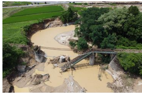
(b) Bridge washout on Banetsu-west Line in 2022
