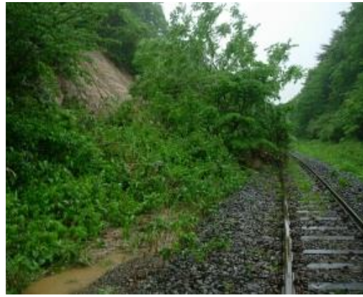
(b) Cut collapse
