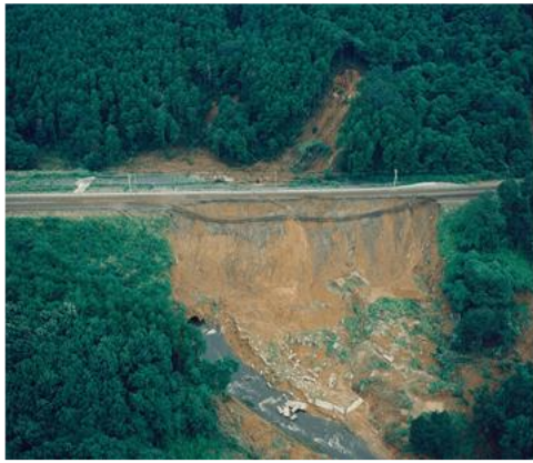
(a) Embankment collapse
