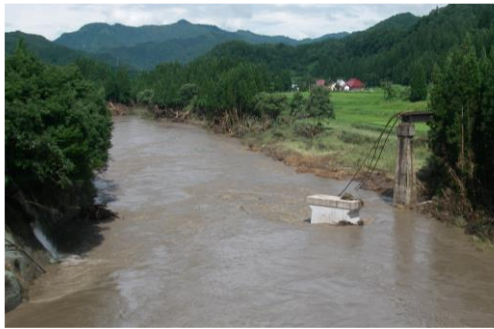
(a) Bridge washout on Tadami Line in 2011
