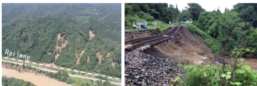
Figure 1: Examples of landslides along railway routes in mountain areas.
