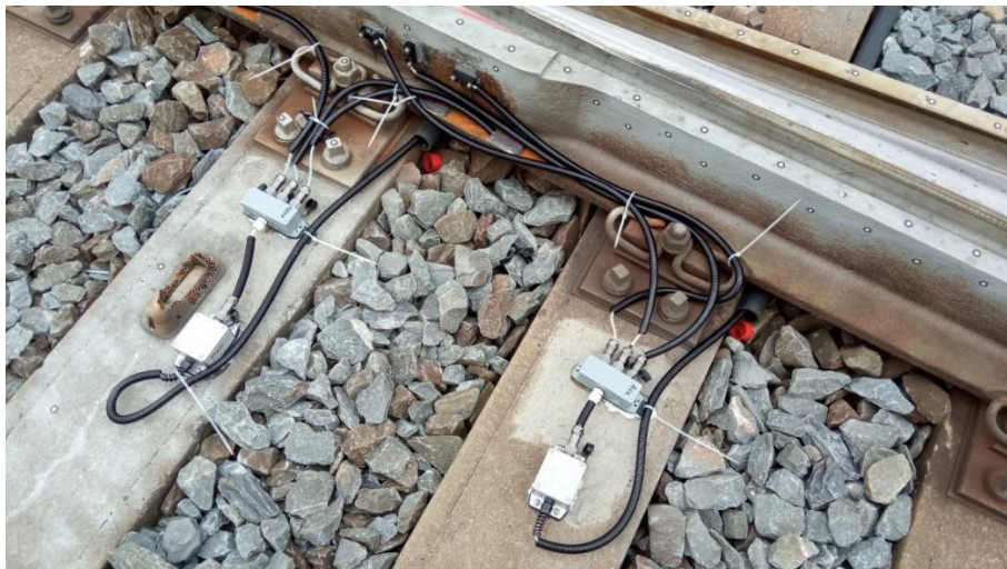
Figure 2: Positioning of measuring devices in the track with the hub and connected sensors.
