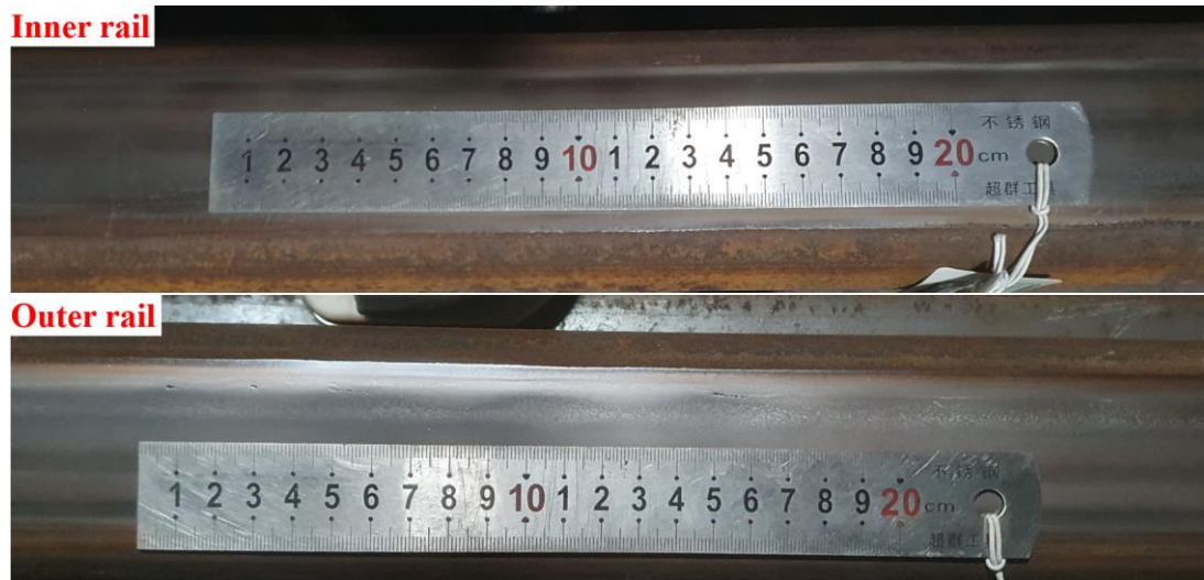
Figure 3: Inspection of rail corrugation in the left line.
